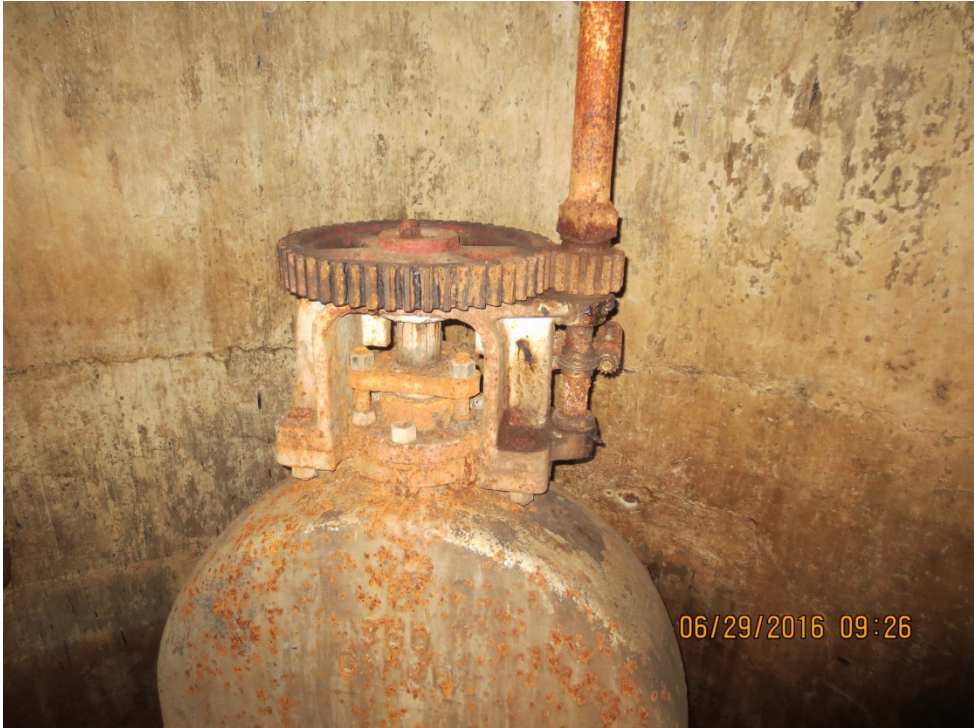
Figure 6: Existing Valve Operator
