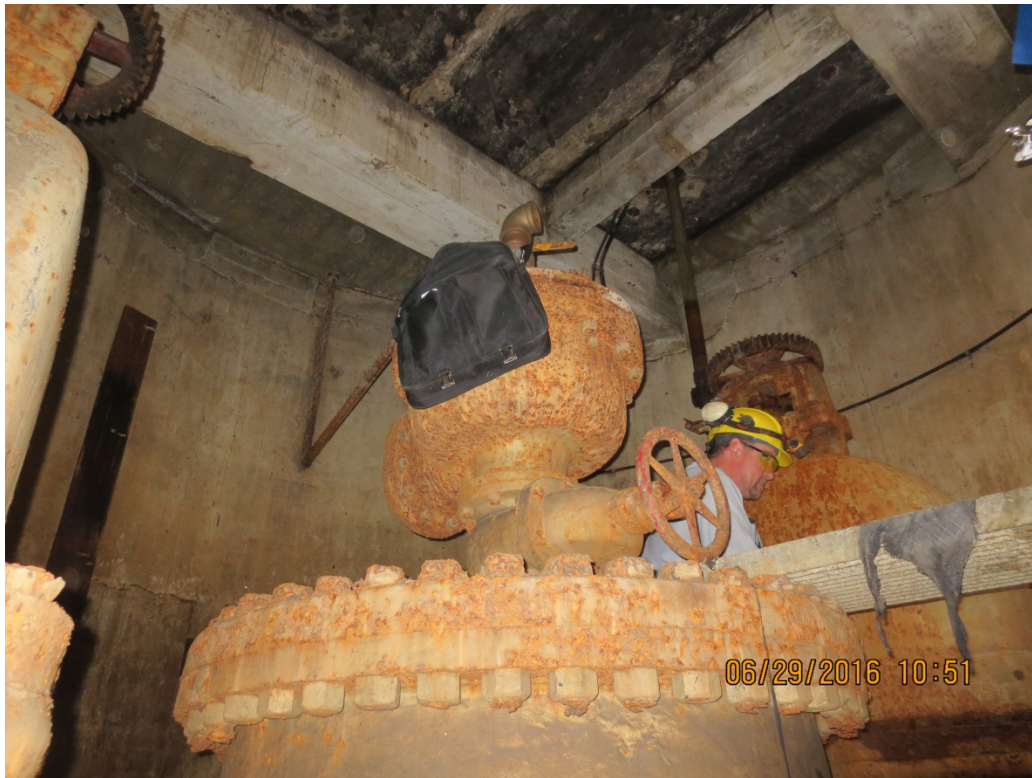
Figure 3 - Existing 200 mm Air Release Valve and 1200 mm Blind Flange
